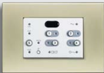
A complete range of devices allows you to program the burglar alarm according to the specific needs of the building to be protected.
